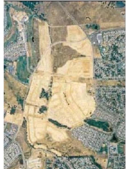
Large residential subdivision under construction in the Upper Deer Creek subwatershed near El Dorado Hills.
