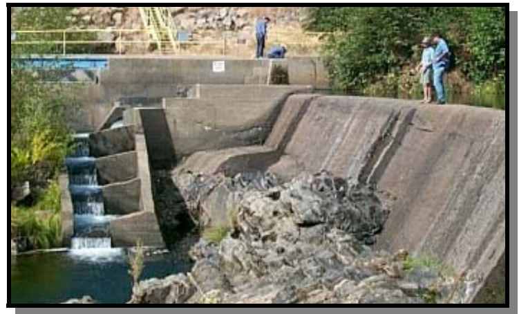
Standing atop Granlees Dam, Fisheries Biologists, Trevor Kennedy (left) and Keith Whitener discuss the improvements made to the fish ladder recently repaired by the Fisheries Foundation of California.
